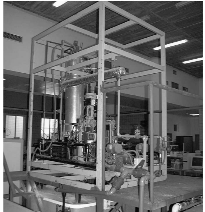
Fig. 1. Pilot plant used to apply the proposed MMMPC.
